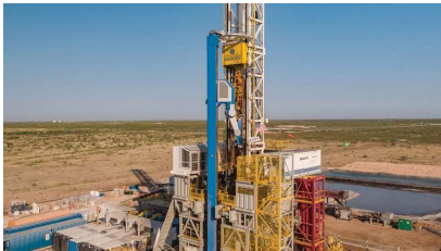
Source: Nabors PaceR801 – JPT Article https://jpt.spe.org/a-robot-takes-over-the-drilling-floor
