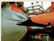
Pipe Failure Due to Sand Erosion (Courtesy Oilfield Wiki)
