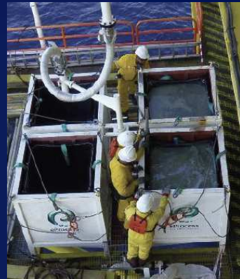
Dewatering Bin Transport Sand Jetting System Malaysia 2015
