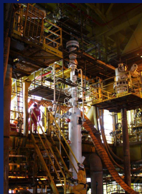
Wellhead Desander, 1500# Solids D98 = 16 micron 600 liter Accumulator
