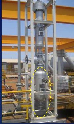
Wellstream Desander Acc. ASME 900#, 108 liter Turkmenistan 2011
