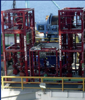
Sand Filter API 10K Australia 2013
