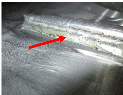
Discoloration (lack of pickling and passivation)
