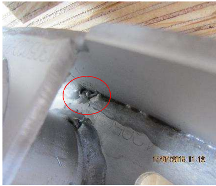
Weld defect (incomplete filled groove)
