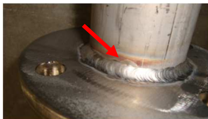
Discoloration (lack of pickling and passivation)
