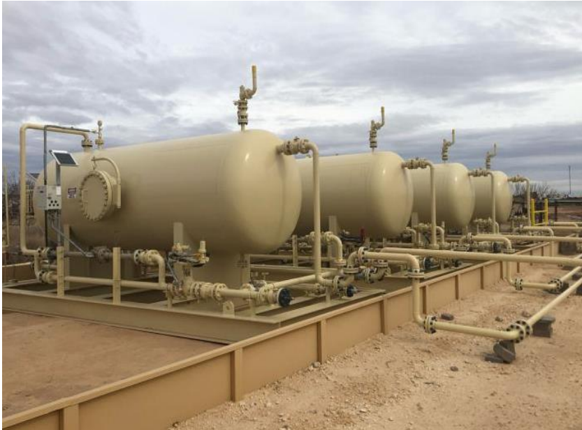
Traditional test separator based well-pad facility
