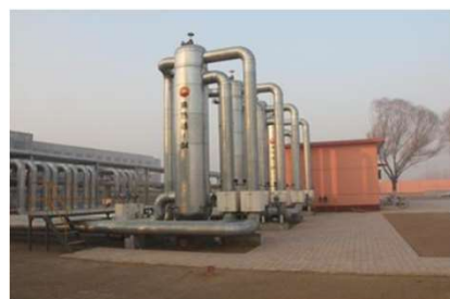
Heat exchanger and geothermal power generation plant
