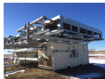
ORC unit installed after repurposing well
